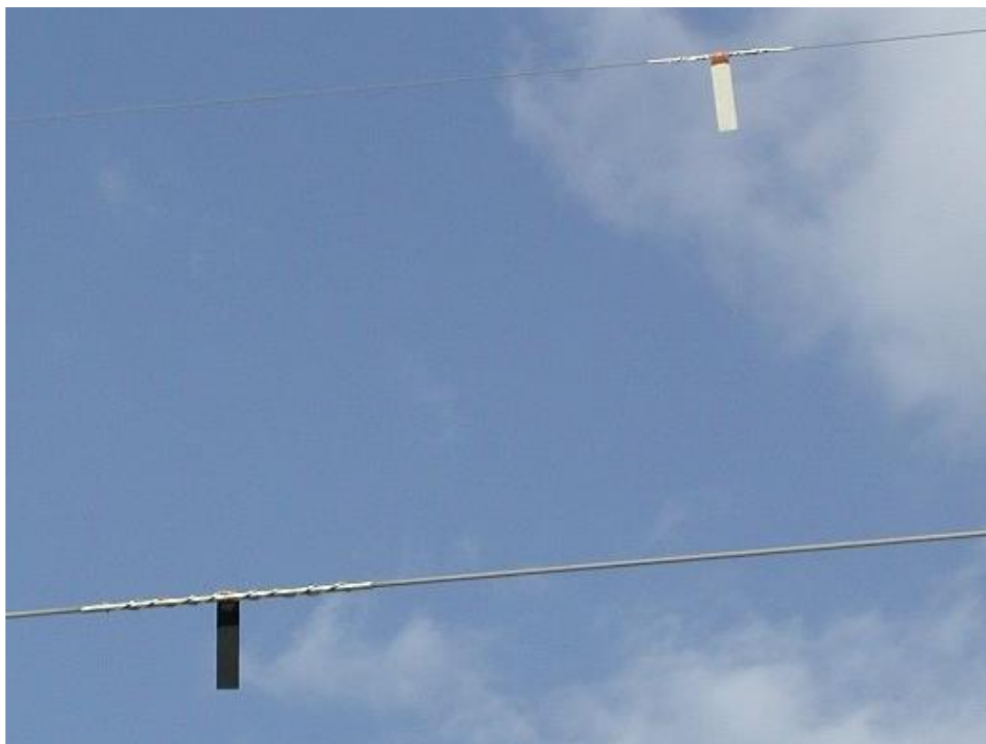
Figure 4: Bird protection flags on high voltage power line in Austria (Photo: H. Herzig).
