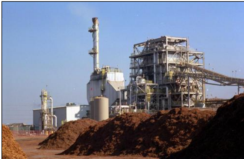
Biomass energy generation facility, California, United States. Photo credit: National Renewable Energy Laboratory
