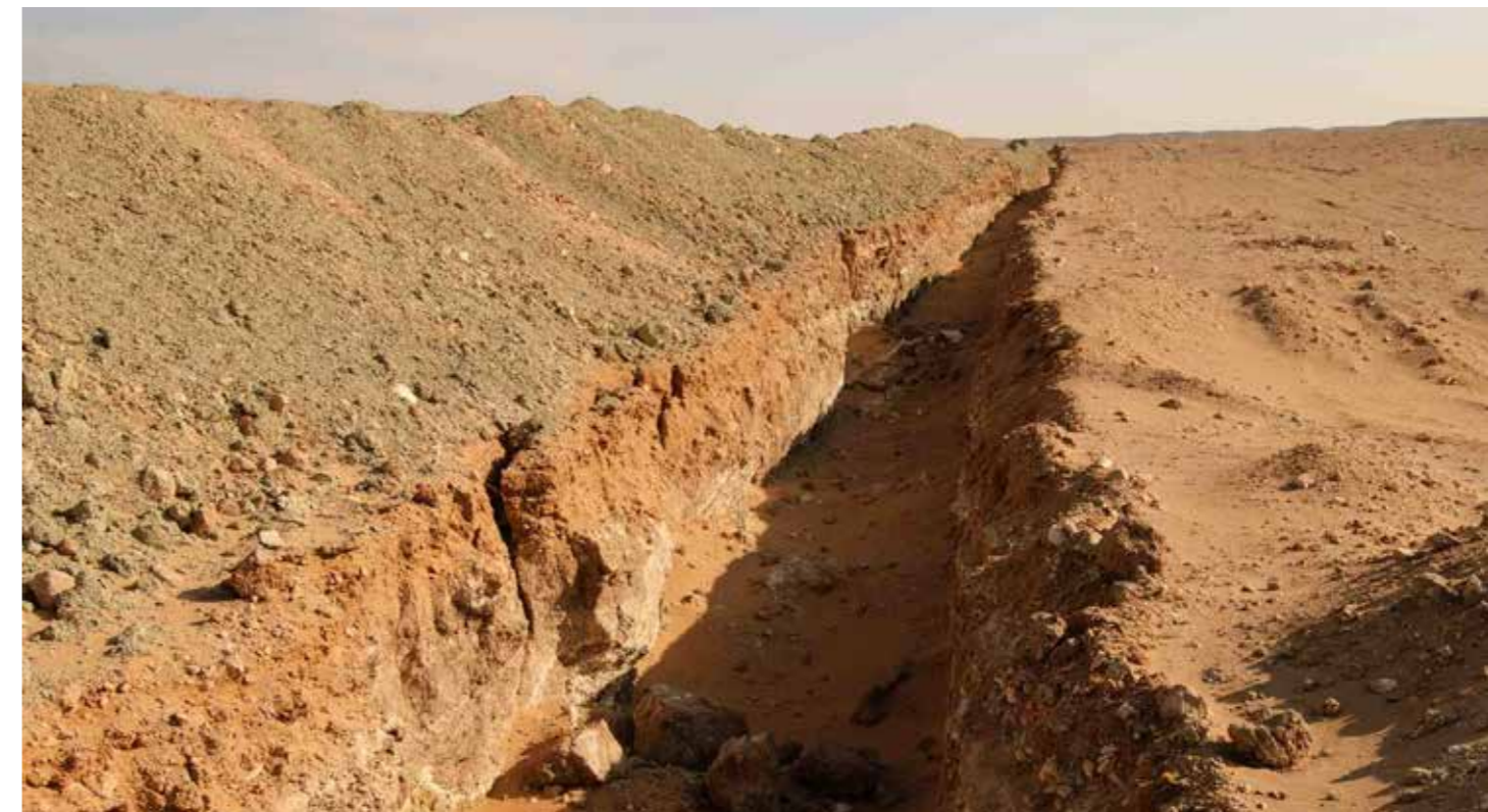
Ditches created during the construction of pipelines or as a measure to prevent vehicles from leaving established roads represent another hazard and potential barrier to wildlife movement. ©WCS/K. Murphy
