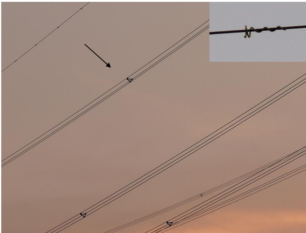
Figure 6. High voltage (380 kV) transmission line with spacers (arrow) to keep individual energised phase conductors in each bundle apart. The single thin wire in the top left corner of the photo is the ground wire (also called neutral or earth wire) that is mostly positioned above the phase conductors. In this case the ground wire has been equipped with small spirals (so called pig tails, see inset) to make this wire better visible to birds (Photo: Bureau Waardenburg).
