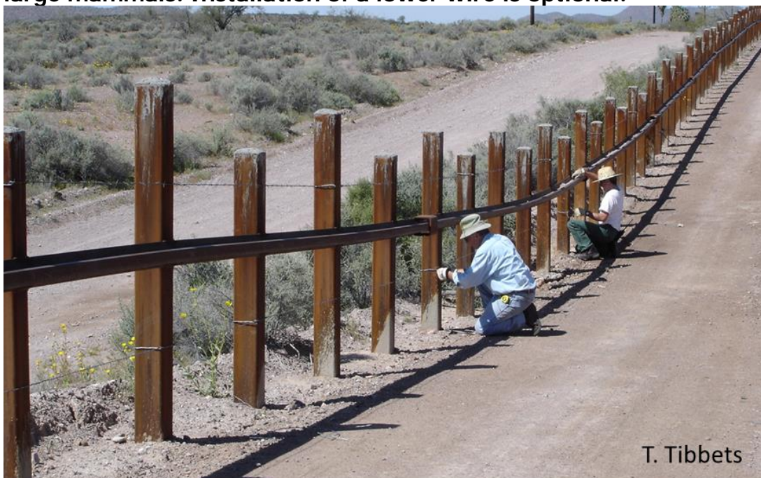
Figure 19. A post on rail vehicle barrier helps to maintain connectivity for large mammals. Installation of a lower wire is optional.
