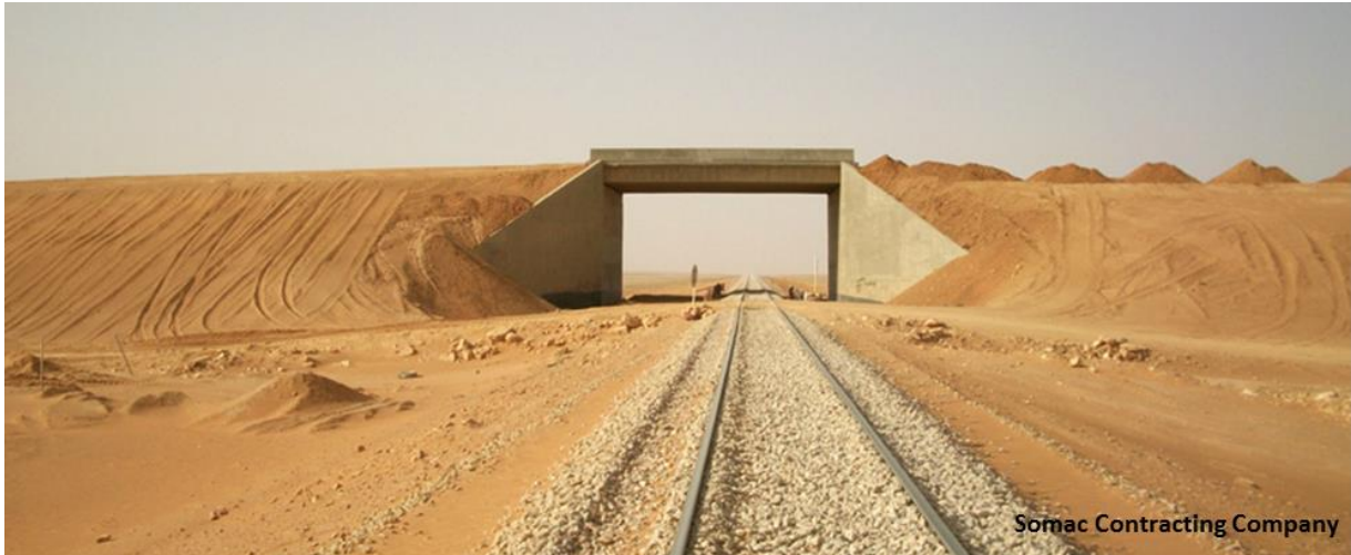
Figure 25. Preparation of an overpass crossing structure for camels across a single track line for a high speed rail in Saudi Arabia.
